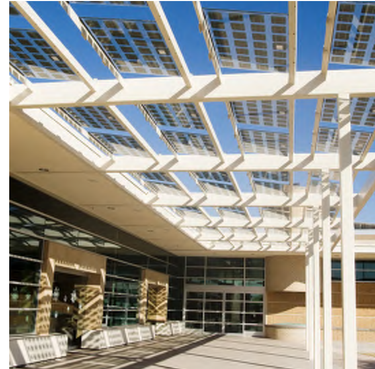
Illustrative Photo: Commercial Facility w/ Solar Array Entry Canopy
